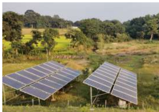
Solar installation, Jharkhand
